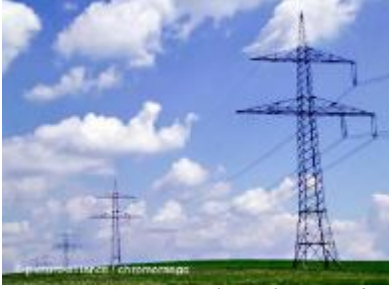
Experts say Germany's electrical supergrid network needs to be made more flexible
